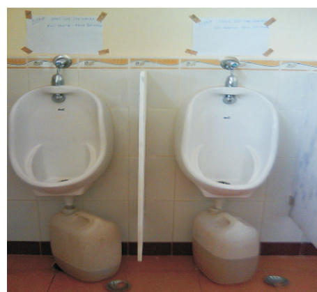
Waterless urinal installed in a male toilet (urine collection)
